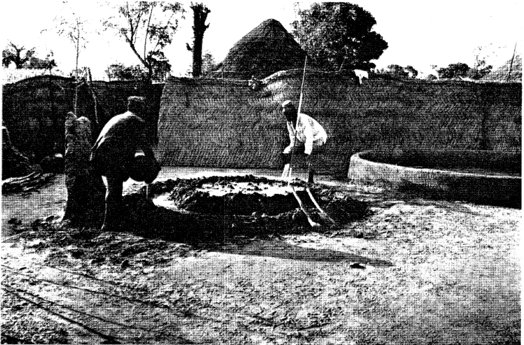
Plate 2 Immigrant labourers repuddle the walls of a hut to build another of which two courses have been laid. The tools include a locally made copy of a European shovel and a wooden club
